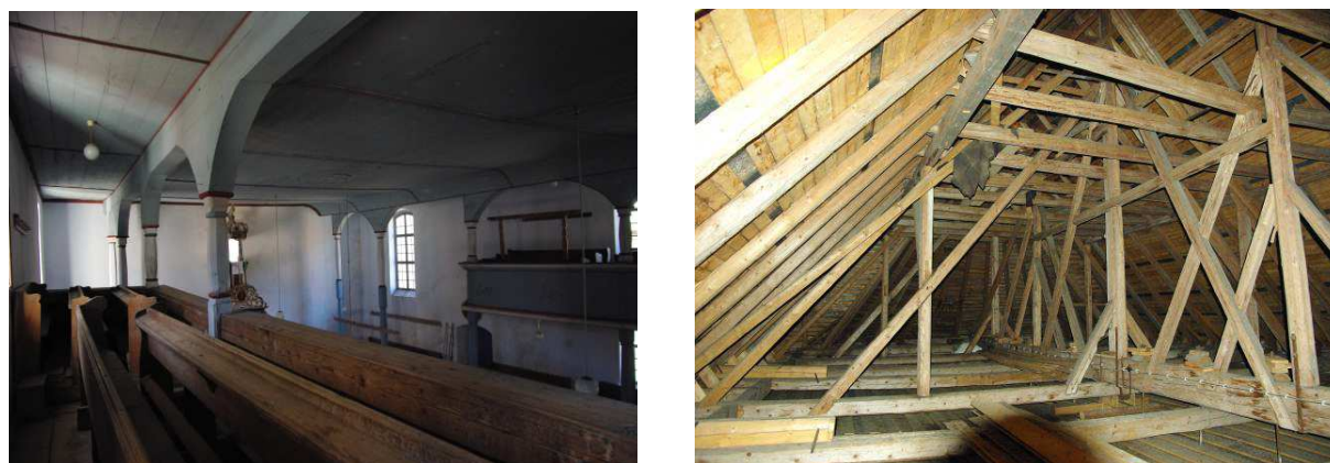
Fig. 6 Visible deflection of ceiling, right view into the under roof space (hanging truss)
