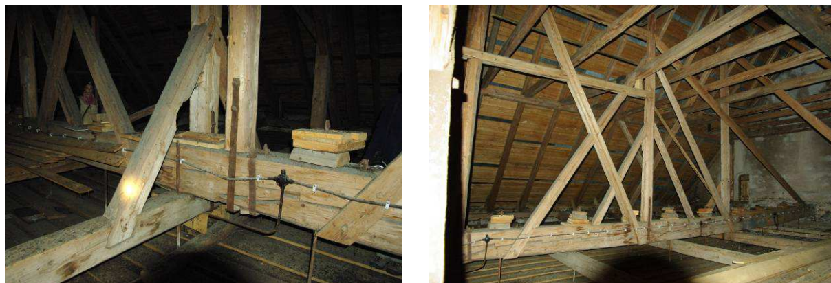
Fig. 8 Left - joint the king-post with a beam grill and extension the lower beam of girder grillage. Right - view to the truss-post ceiling.
